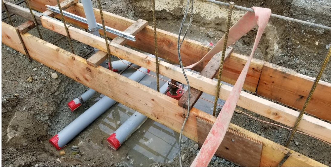
Electrical Underground Sleeves
